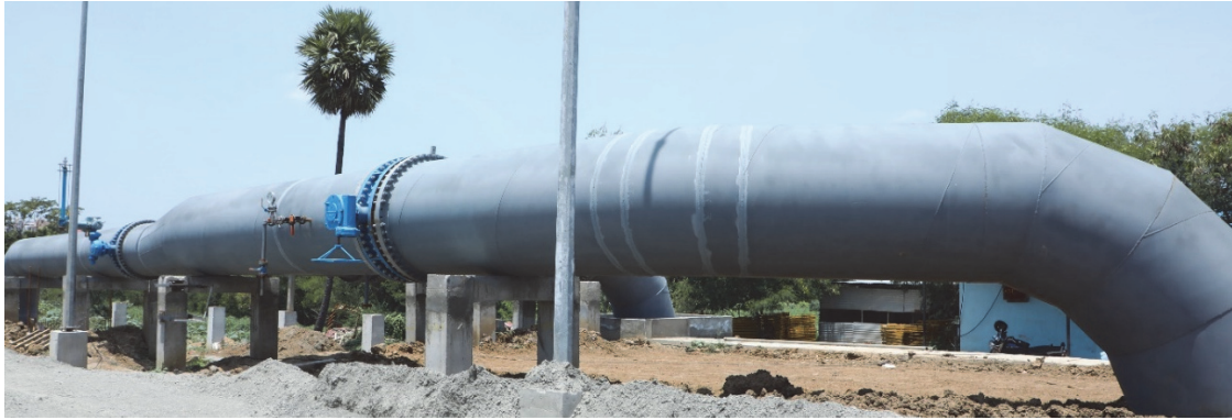
Figure 2 – Reclaimed water pipeline (photo taken in August 2019)
