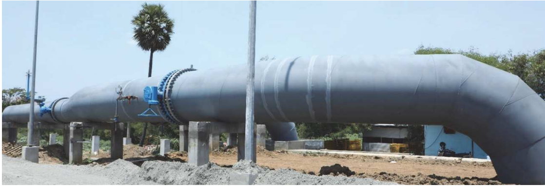
Figure 2 – Reclaimed water pipeline (photo taken in August 2019)
