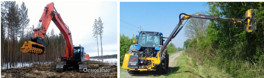
Fig. 3. Mulchers mounted on the boom of an excavator and a manipulator of a wheeled tractor.
